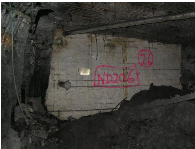
Figure 26 above shows stowage against goaf stopping impeding access.
