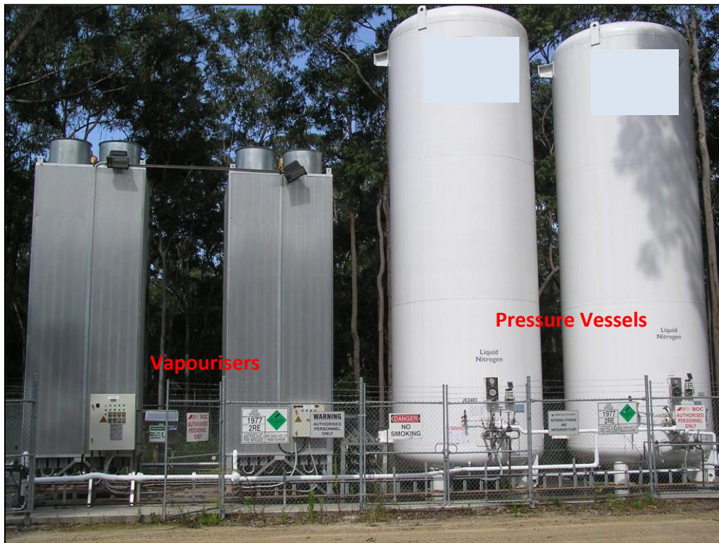
Figure 28: Ambient air vapouriser
