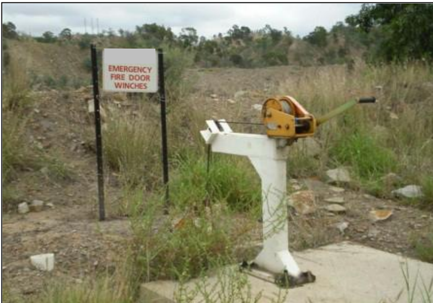
Figure 35: Surface located winch to activate door
