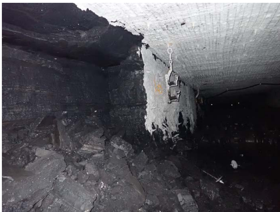
Figure 3 – Failed section of rib (SinNot-2018/00638).
