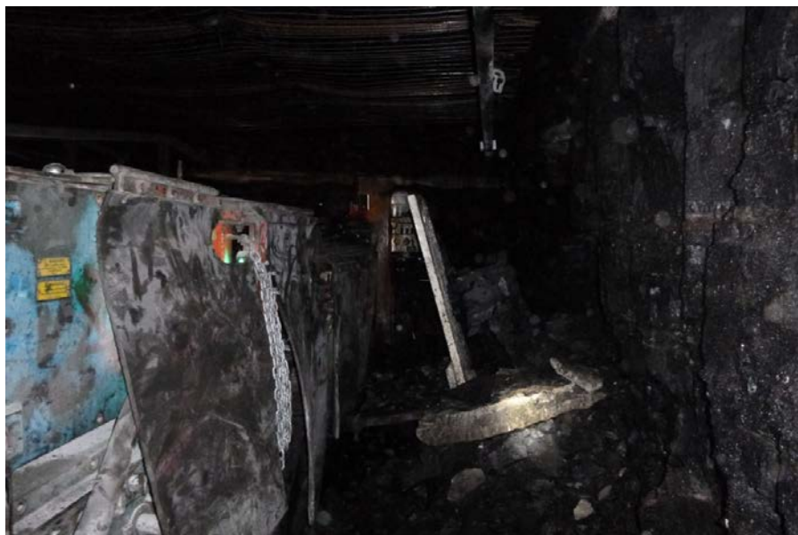
Figure 3 – Rib failure striking platform. Note that the platform has been rotated back down towards the normal operating position (SinNot-2018/00854). Photo courtesy of the mine.
