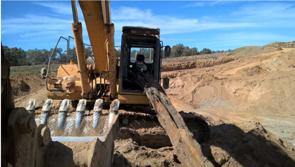
Figure 2: While lifting a log with an excavator, the log slipped and entered the cabin front window. (SinNot-2017/01622)
