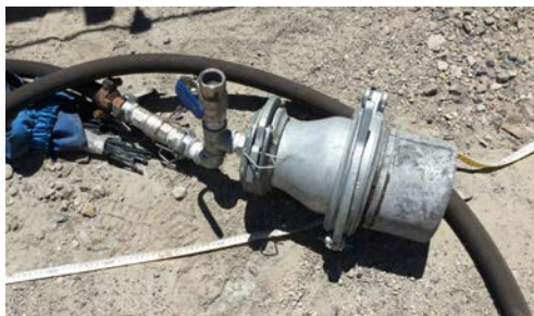
Photo 2: Ferrule, blanking plug and test fittings
