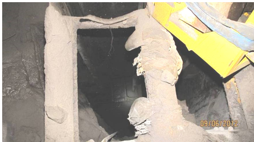
Figure 11: The steel RSJs protruding at shaft access level and the gaps with the view to the base of the shaft 14 metres below. The end of the yellow steel weight basket is visible lodged on steel RSJs and one of the blue coloured fibre slings.
