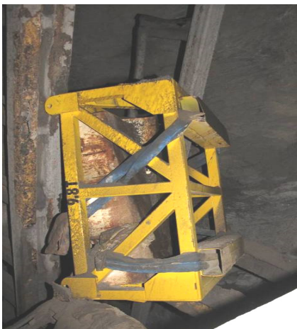
Figure 10: The weight basket lodged vertically on its end on the steel RSJs at the shaft access level. There were only two 3 tonne weights remaining in the weight basket
