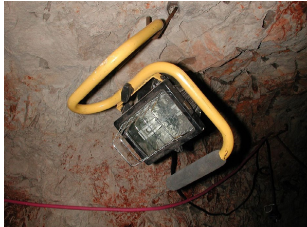
Figure 147 - Protected light fitting, floodlight.
