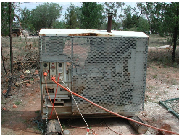
Figure 129 - 415 volt (3 phase) generator
