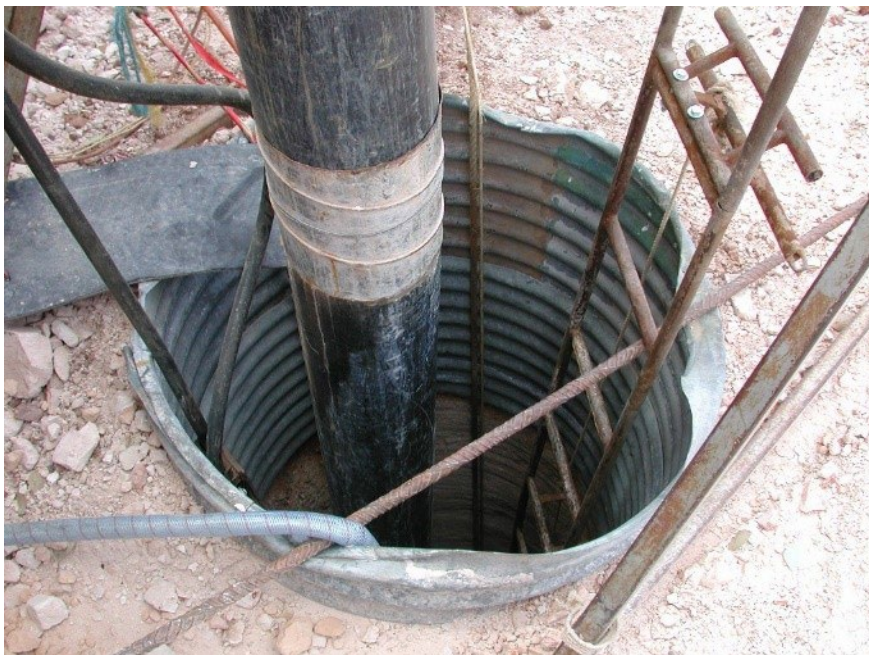
Figure 15 - Poor surface layout resulting in restricted shaft access
