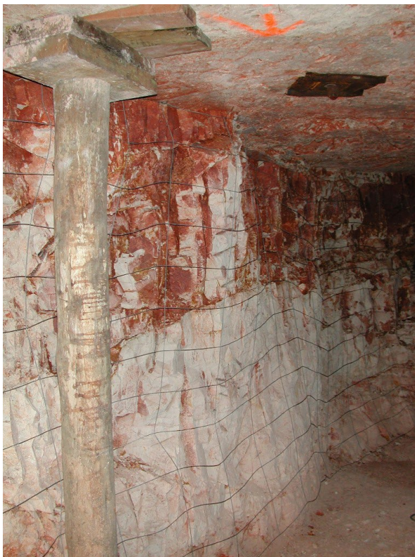
Figure 71 - Pillar support using wire netting is ineffective as the mesh is too large
