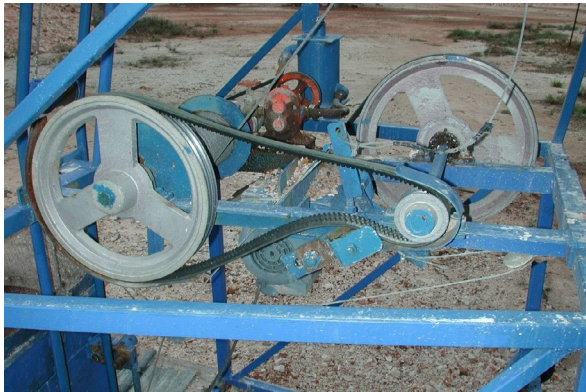
Figure 8 - Exposed belts and pulleys on a hoist
