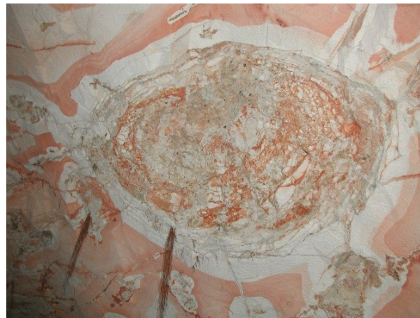
Figure 37 - Blow in the roof of a mine drive
