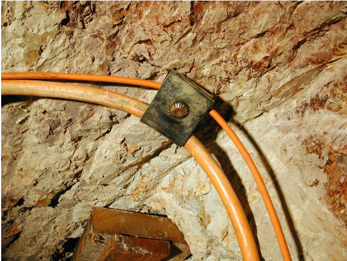
Figure 143 - Electrical cable secured to drive roof with rubber and a steel pin.
