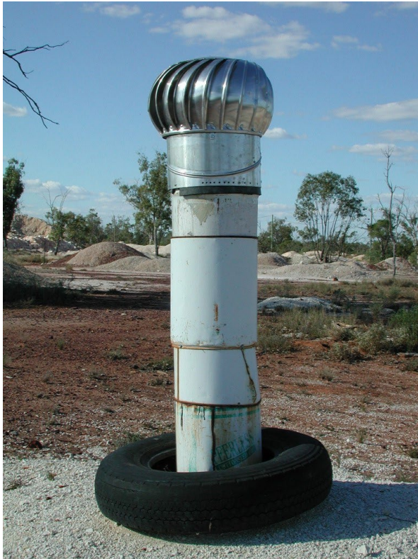
Figure 85 - Ventilation fan over and auger hole
