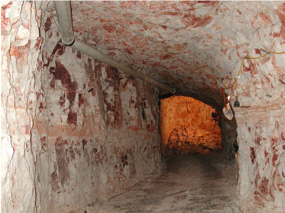
Figure 88 - Ventilation tubing hung from a walk of drive supplying fresh air to the working face
