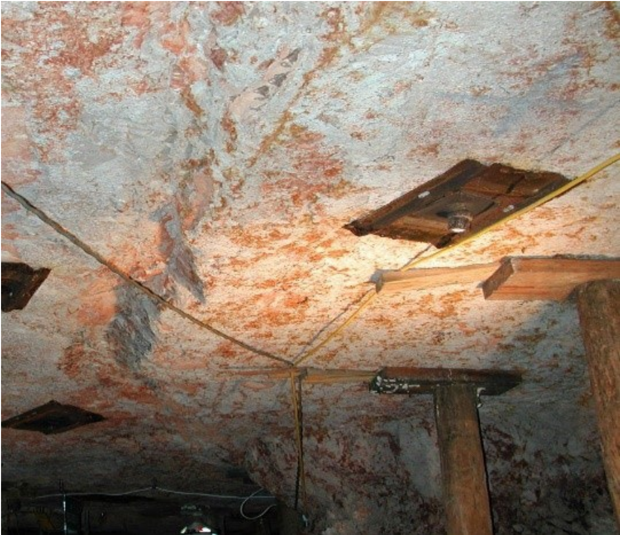
Figure 53 - Rock bolts and props being used in a drive for roof support either side of a fault
