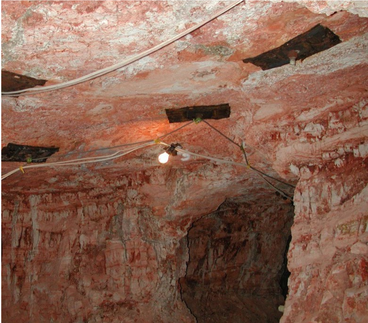
Figure 68 - Concentration of rock bolts above a drive intersection
