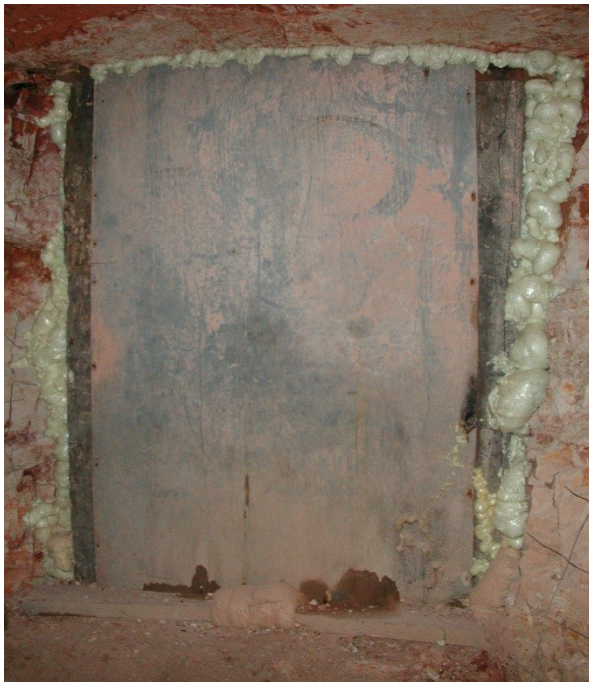
Figure 92 - Plywood ventilation barrier across an old drive
