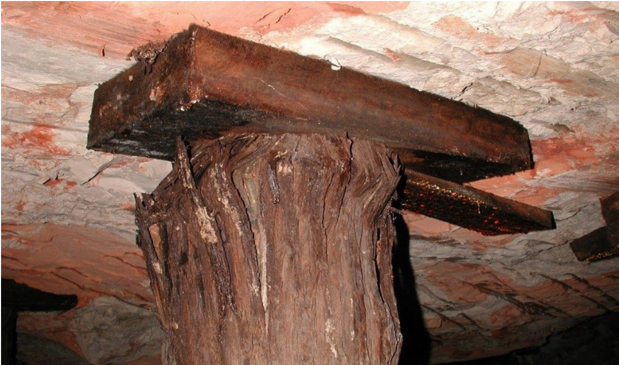
Figure 61 - Prop showing substantial pressure
