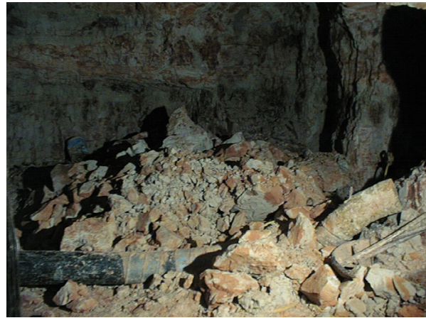
Figure 51 - Rock that fell from the roof as a result of discontinuities and inadequate secondary support
