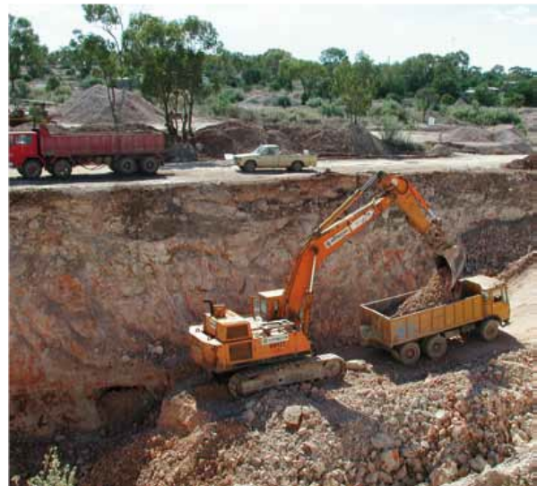
Figure 95 - A 45-tonne excavator loading a 10 cubic metre tip truck. Standards require that there to be a bund wall around the excavation edge.
