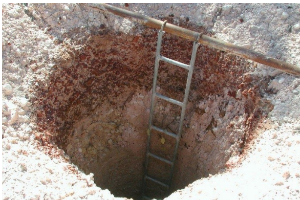
Figure 11 - Hazardous shaft collar with loose gravel
