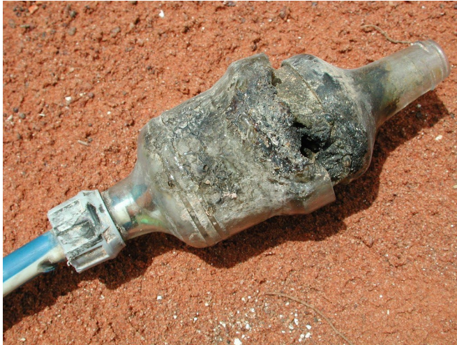
Figure 127 - Electrical cable burnt out after contact with condensation moisture in a mine shaft.
