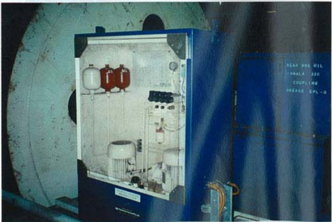
Modern drum winder drive and brake arrangement showing high and low speed brakes, hydraulic power pack and cycle meter
