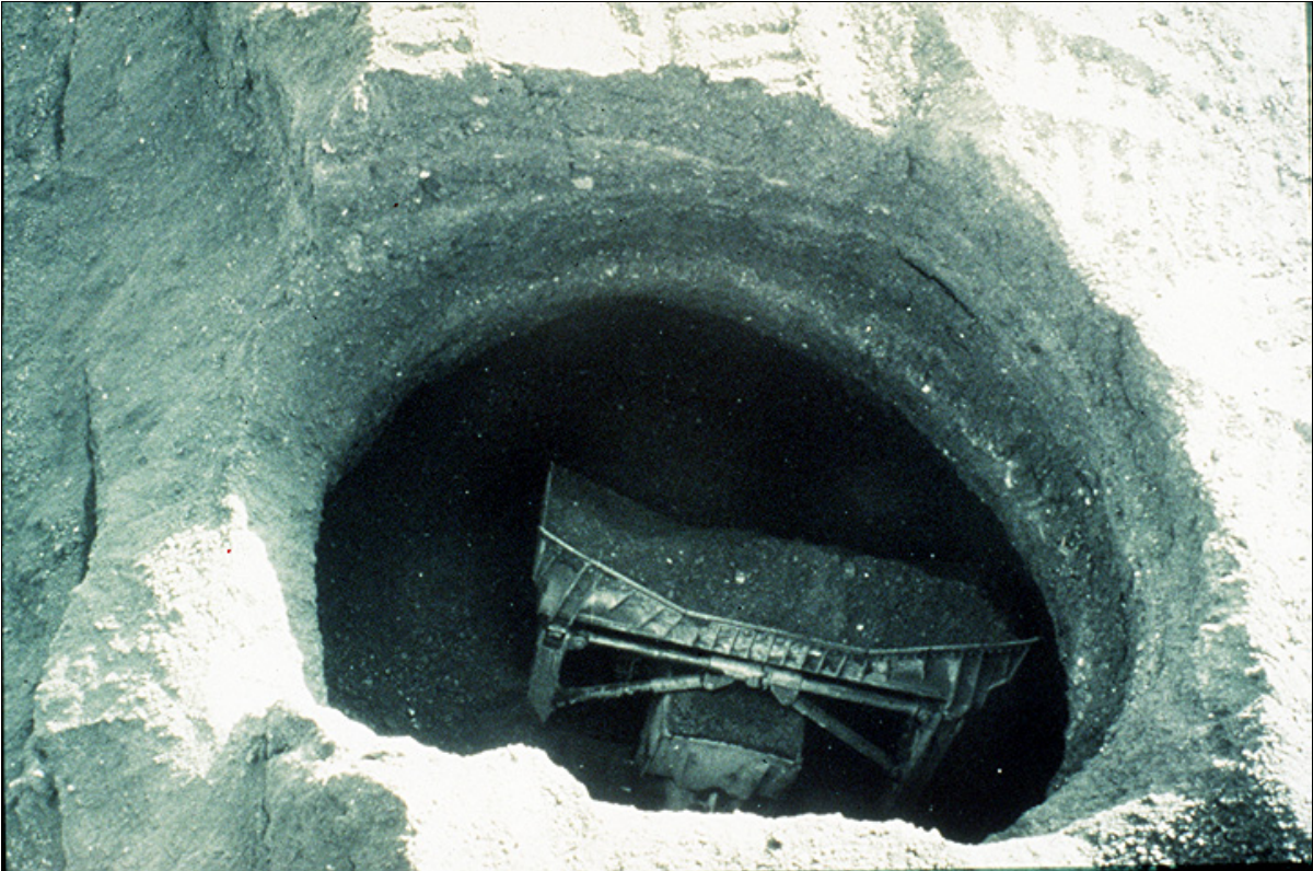
Figure 4. The stockpile dozer has fallen backwards into a draw down point following the collapse of bridging. Note the thickness of the bridged material.
