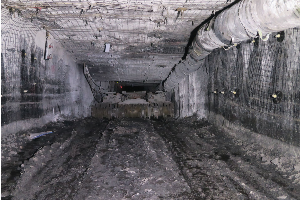
Figure 4 Front view of CM04 after the incident
