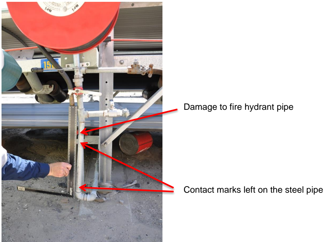
Figure 6 – Damaged fire hydrant at pan 150 CV003 conveyor.
