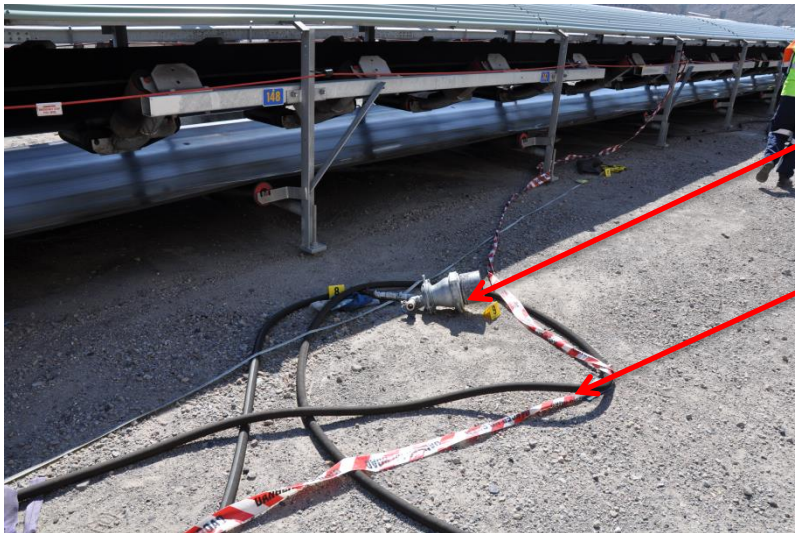
Figure 5 - Incident scene adjacent to conveyor CV003 at pan 148.
