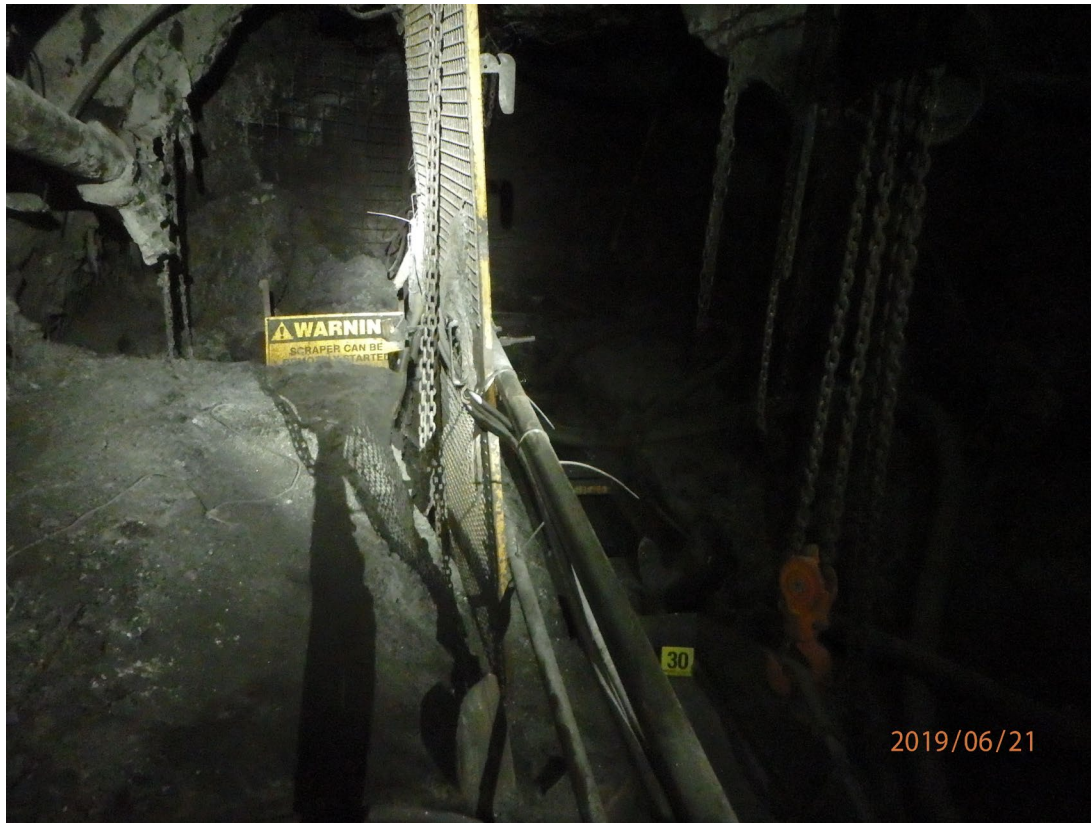
Figure 16. The compromised safety rail height and warning sign partially covered
