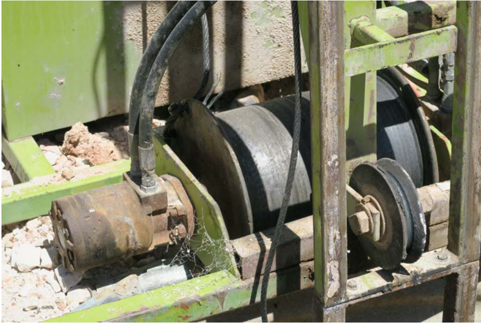
Figure 7: Hoists drum and cable.
