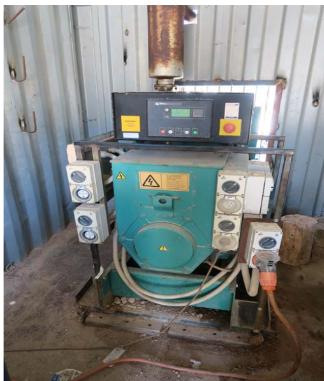
Figure 12: The generator that powers the electric motor to the hydraulic system and underground lights.
