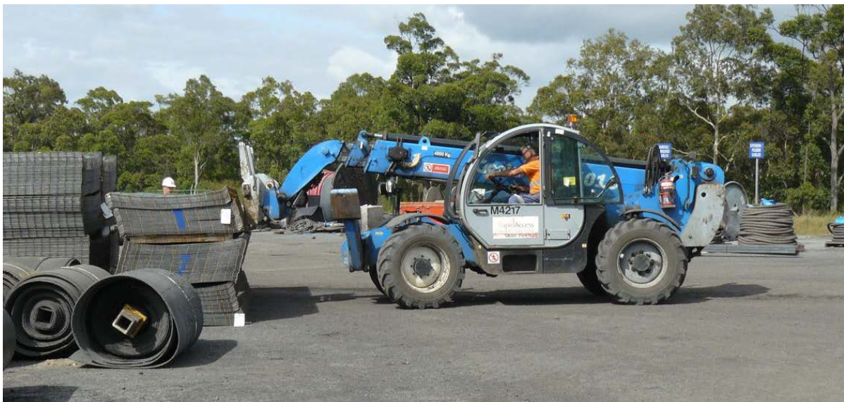
Figure 6: The telehandler that was being used to unload the mesh when the truck driver was injured.
