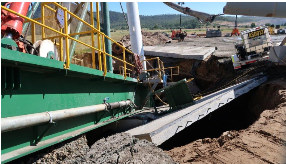
Figure 1: Fan shaft collar collapse
