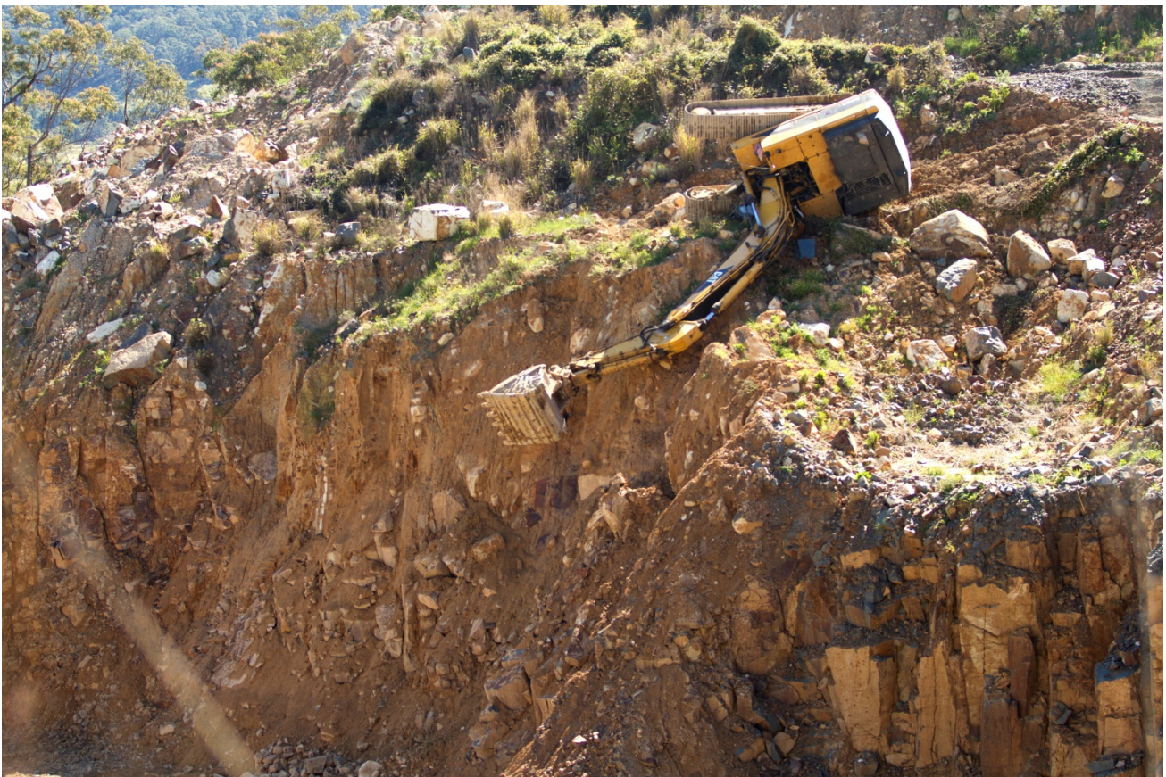
Image 1: Resting position of excavator at top of quarry face - Photograph by Investigation Unit
