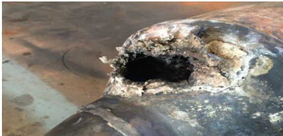
Fig. 2 Close up of where molten stainless steel sintered metal core has burnt through steel casing of DEF.
