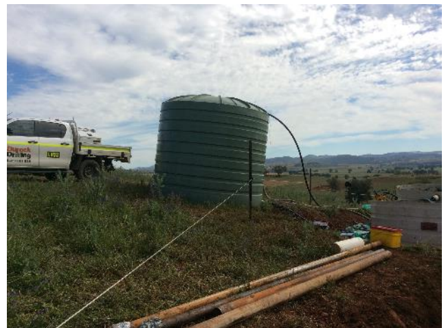
Figure 6 Water storage tank for drilling operations
