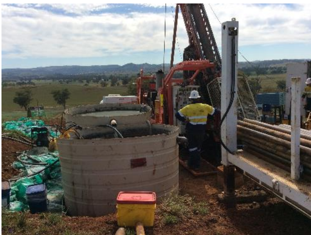
Figure 5 Aboveground sumps for drilling water management
