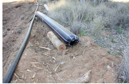
The piece of wood that was placed in the pipe was found at the scene next to a sheared piece of the pipeline.
