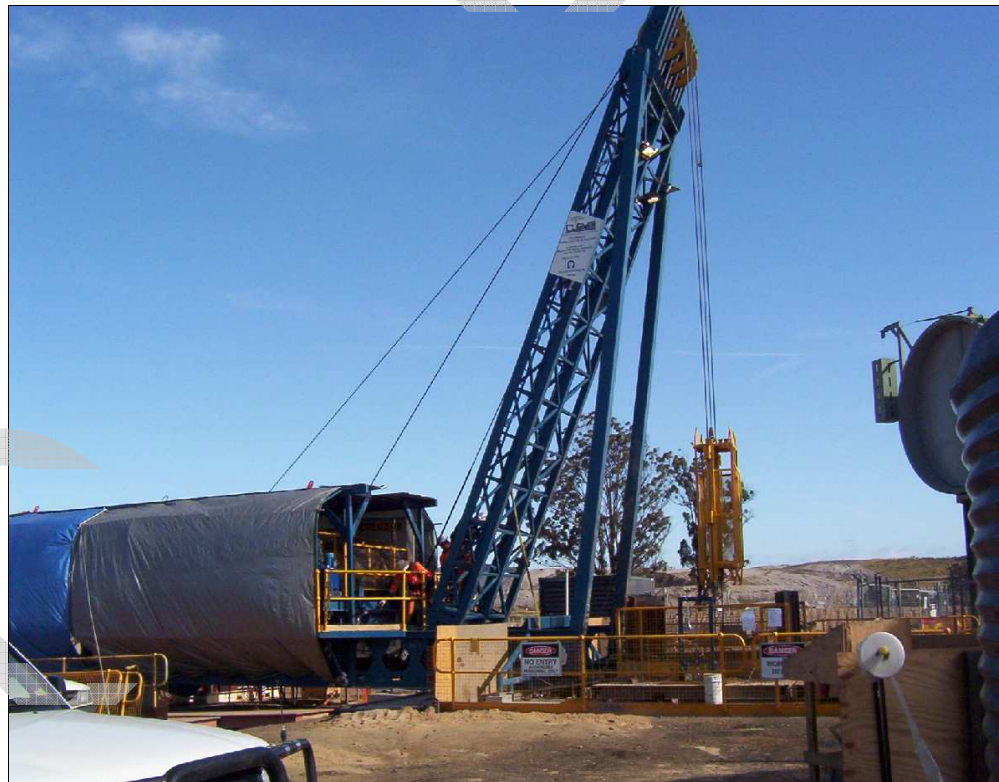
Shaft sinking winder
