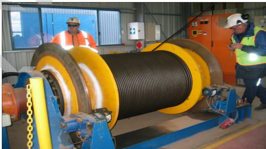
Drum of single rope shaft winder
