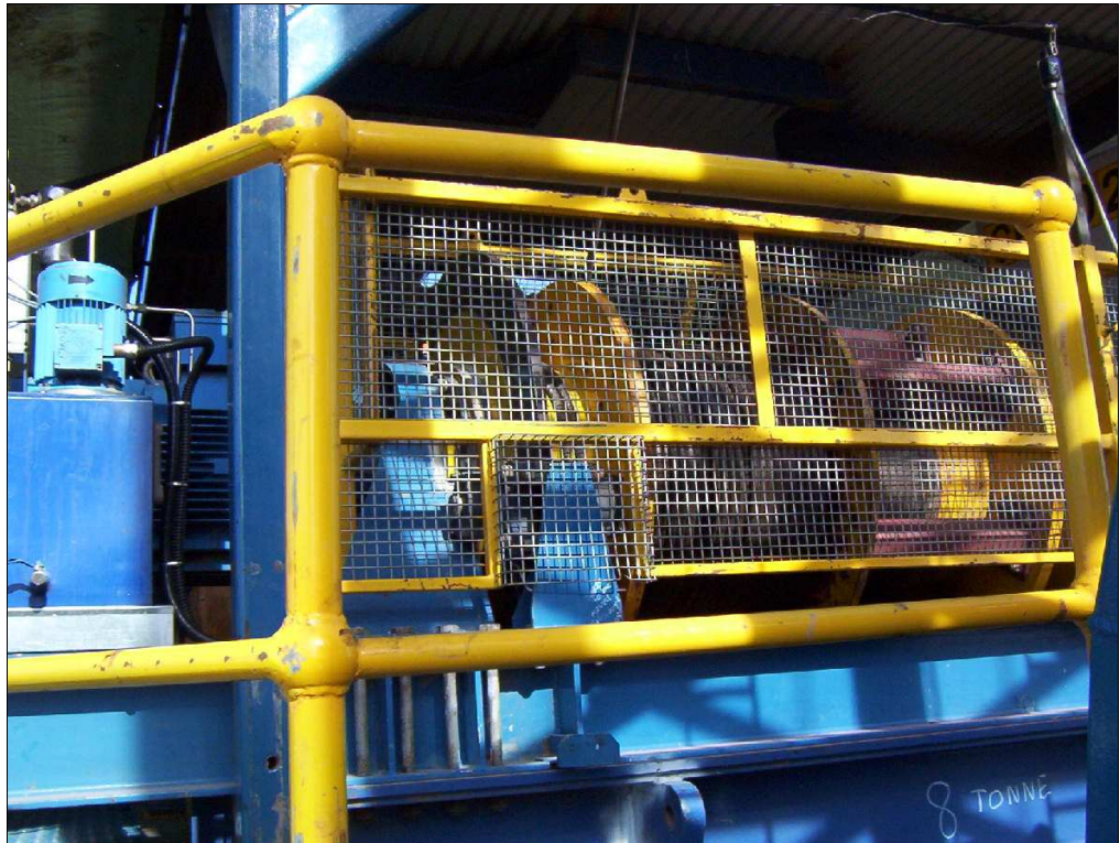
Cable drum of mobile shaft sinking winder
