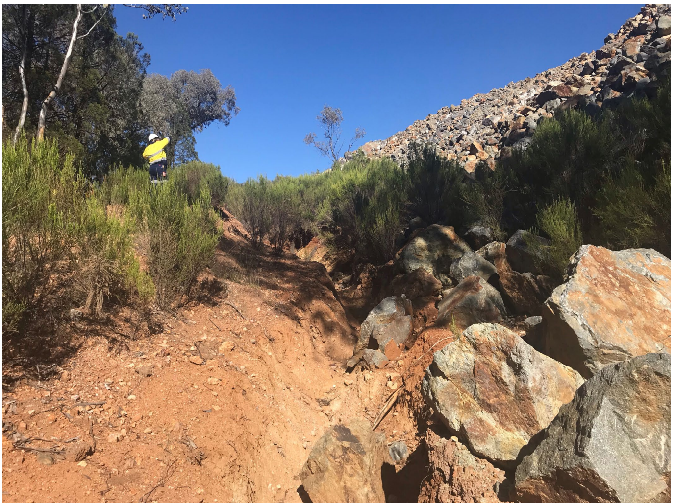
Figure 4 – Erosion at base of tailings dam wall - western NSW
