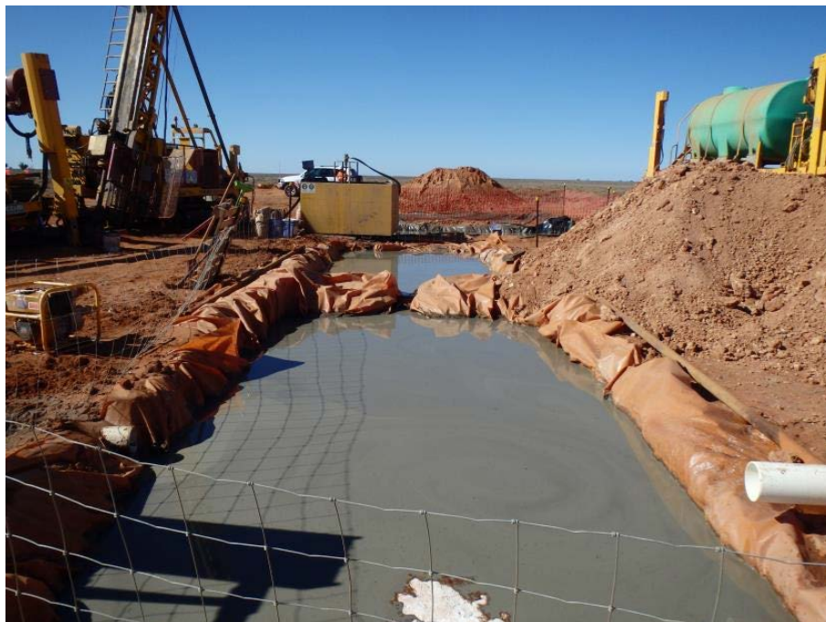
Figure 8 Inground sumps lined and fenced
