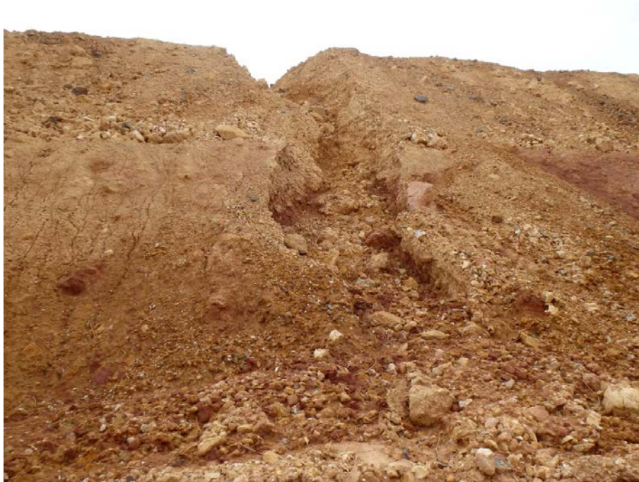
Figure 1 Large erosion scour on a tailings dam buttress wall
