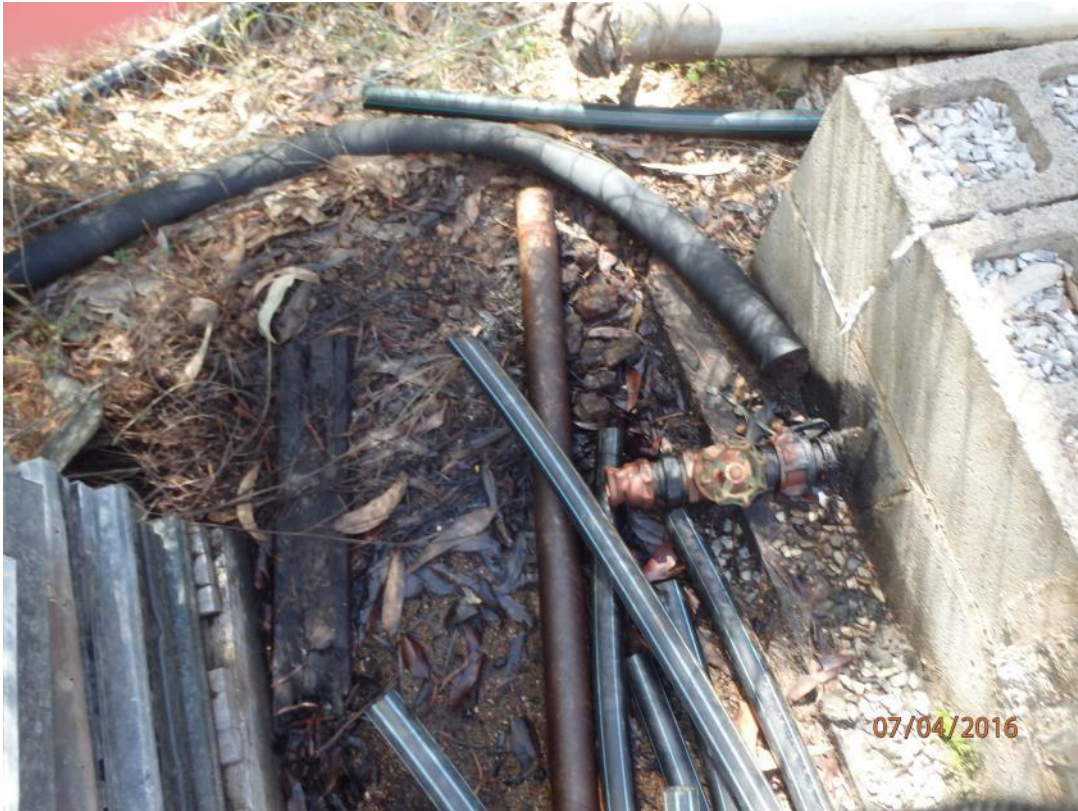
Photo 3 – Bund drain left open discharging potentially contaminated water
