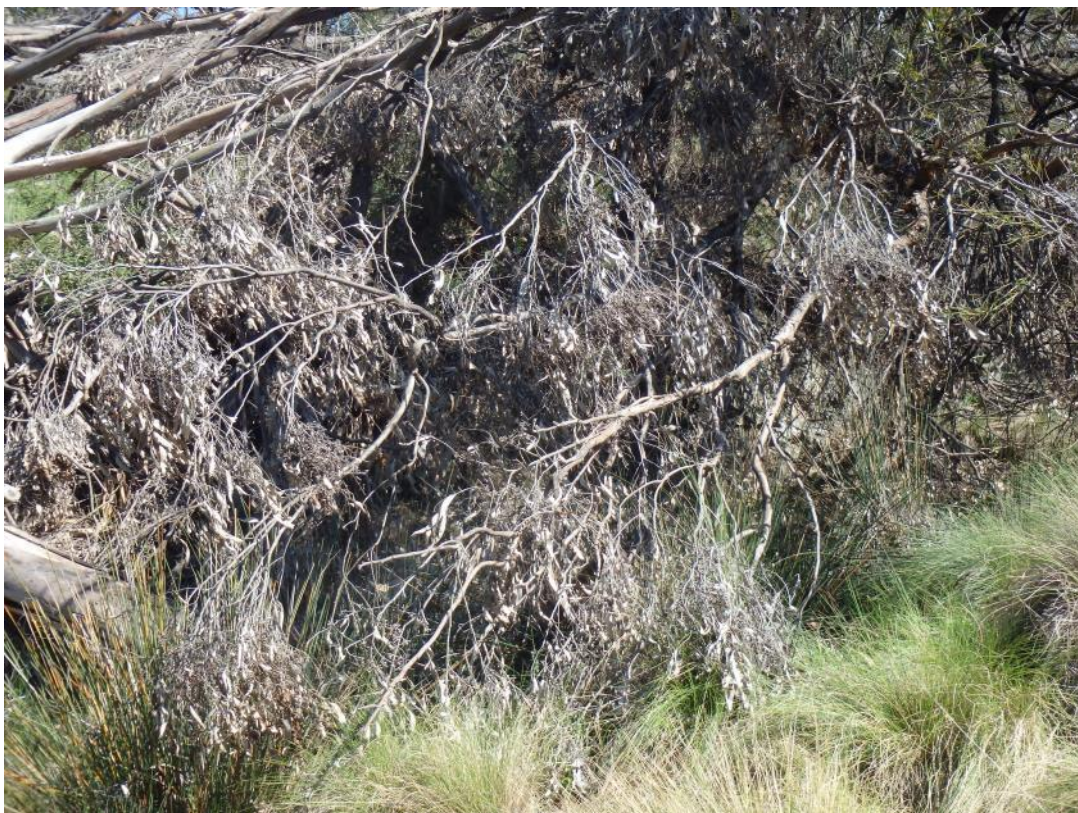
Photo 8 – Fallen tree blocking the grassed spillway on a sediment dam
