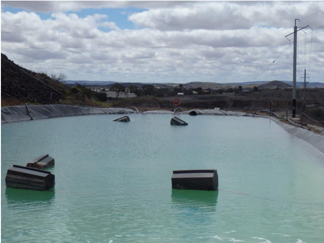
Photo 7 – Inadequate dam wall construction with no operational freeboard and a noticeable low point in the dam wall
