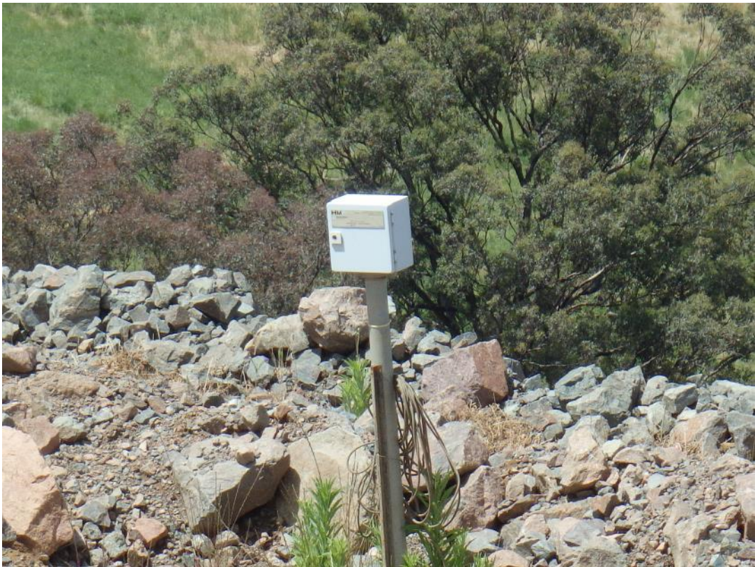
Photo 10 – Example of automatic monitoring piezometer installed on a dam wall
