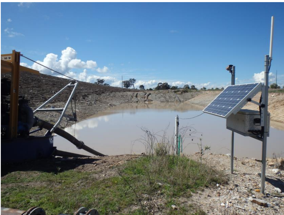
Photo 12 – Example of solar powered automatic water level sensor and webcam installed on a sediment dam
