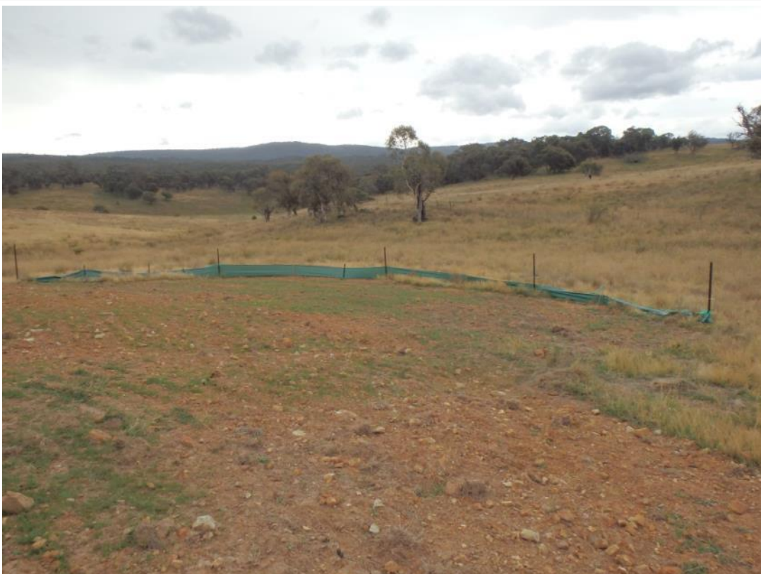
Photo 2 – Sediment fencing in need of maintenance on a drill site
