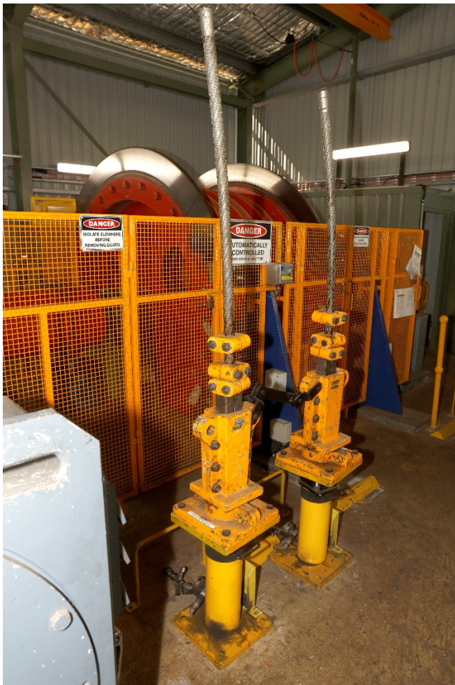
Figure 4. Guide rope tensioning system for cage guide ropes 1 and 2.
