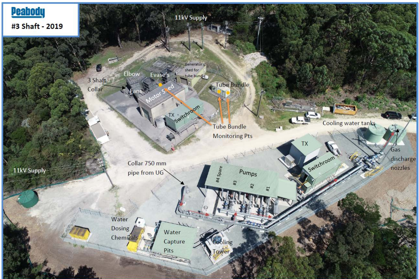
Figure 28 Surface fans and gas drainage plant infrastructure
