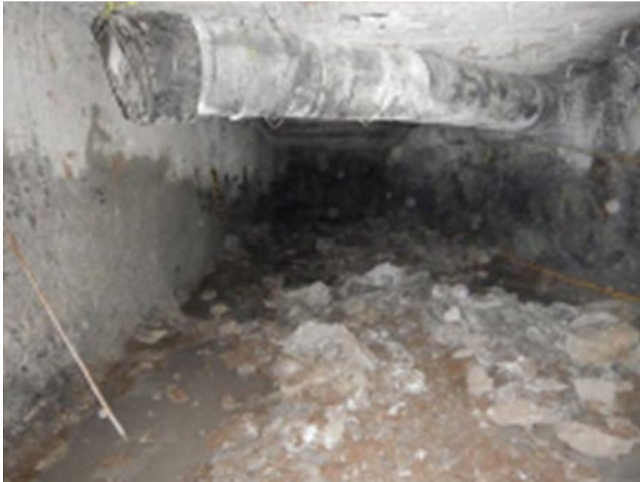
Figure 2 Looking inbye from the bulkhead seal site following the catastrophic failure
