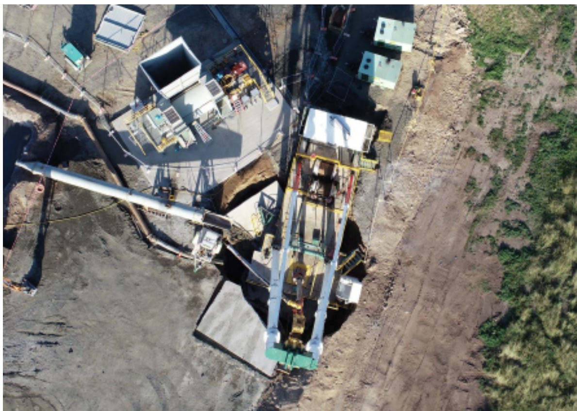
Figure 4 An aerial view of the shaft collar collapse
