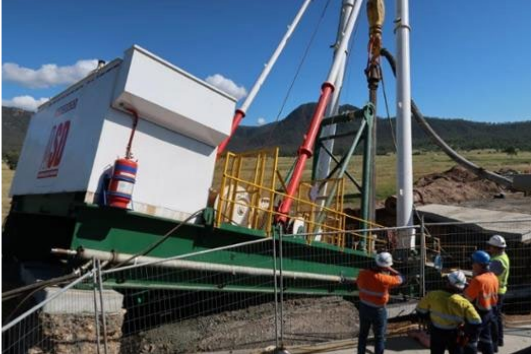
Figure 3 The blind boring drill rig operated by Australian Shaft Drilling Pty Ltd partially sunk in the collapsed shaft
