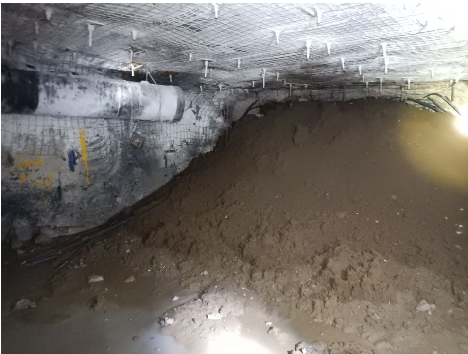
Figure 1 The bulkhead seal location after the catastrophic failure
