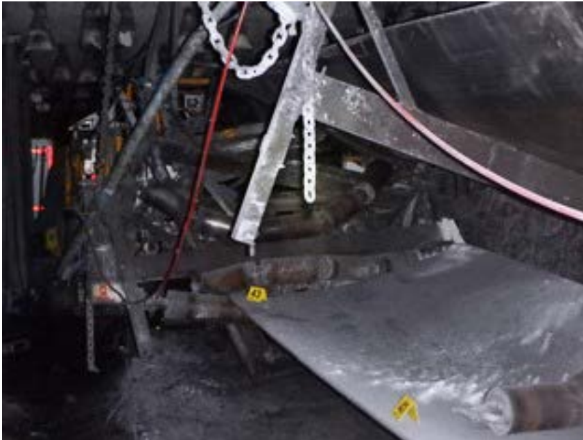
Figure 4 - Damaged conveyor structure outbye of bootend looking inbye.
