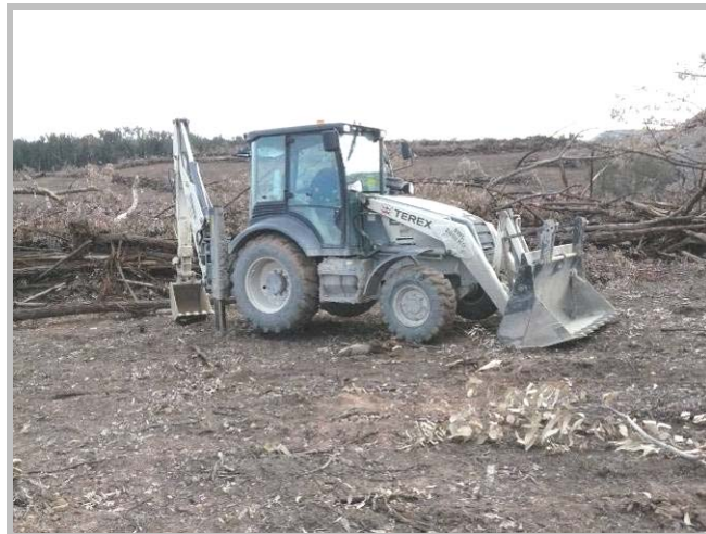
The photo shows the backhoe position in relation to the pile of wood.
