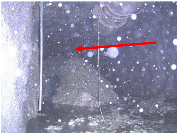
Photograph of the area at the base of the VR5B ventilation shaft.
