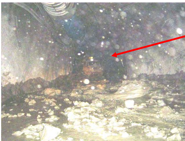
2 nd Photograph of the light vehicle bogged in the inrush material below VR5B shaft.
