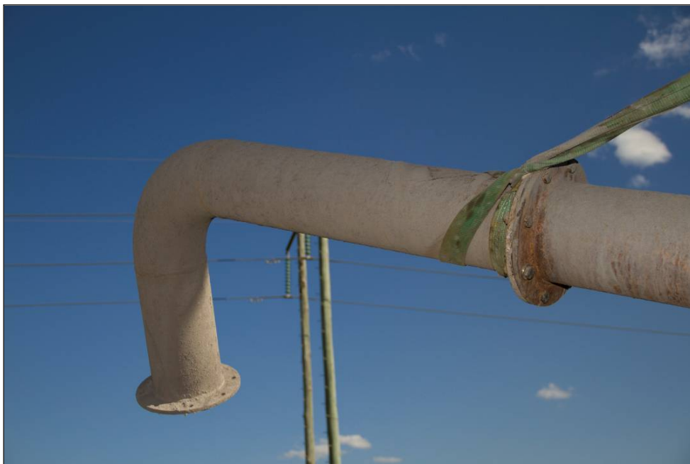
Figure 12. 90 degree elbow on the end of the air discharge line.
