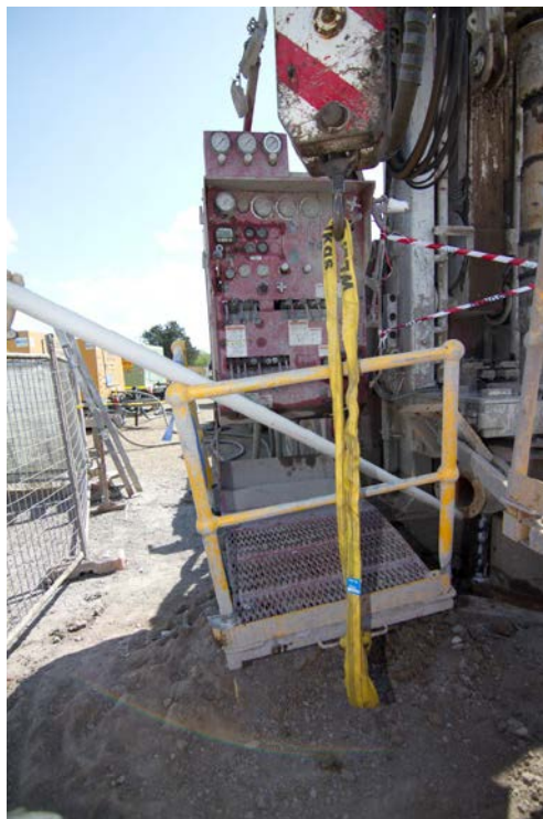
Figure 10. The likely final resting point of the driller's platform. The air discharge line is represented by a white polyethylene pipe.
