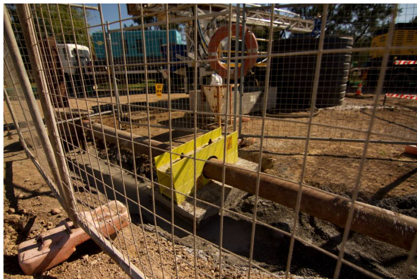
Figure 14. Air discharge line anchor required post incident.
