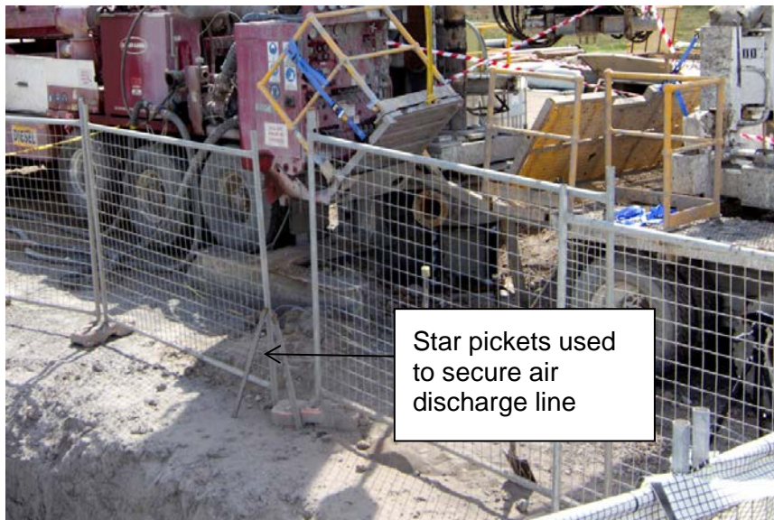
Figure 13. Borehole 4 scene depicting star pickets and fencing wire used as an air discharge line anchor.
