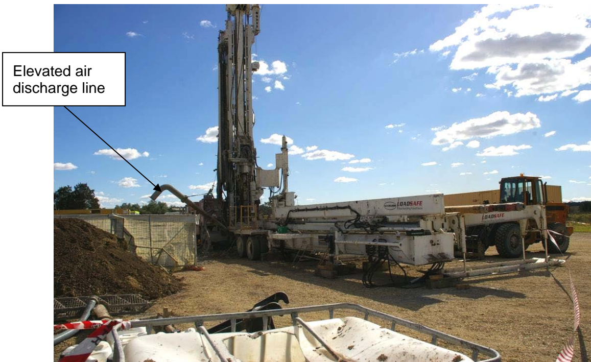
Figure 7. Silver City Drilling drill rig at Borehole 4 post incident.
