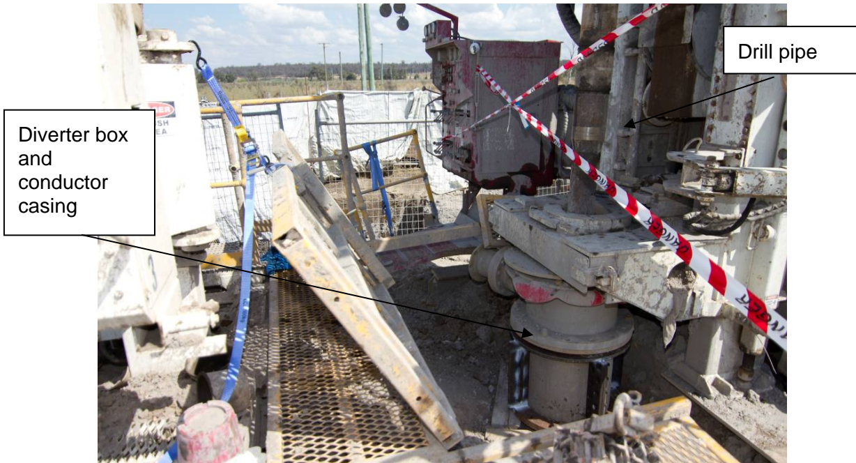
Figure 11. The conductor casing being supported by a steel bracket and the drill string.
