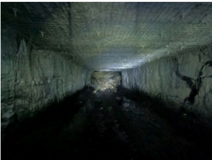
Picture 1. Debris after roof failure
