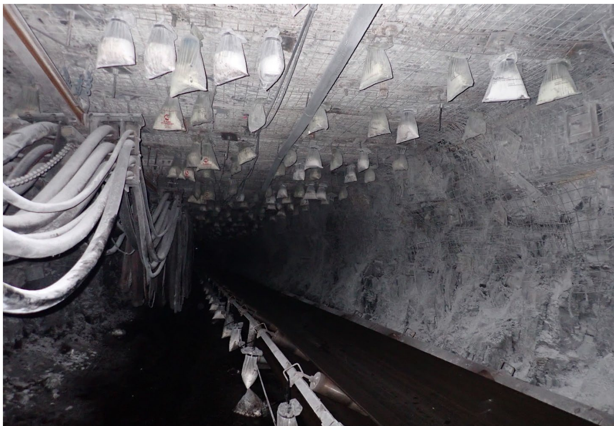
Image 8: Example of a poor standard of installation of a Fixed concentrated barrier in an operational Longwall panel face zone.
