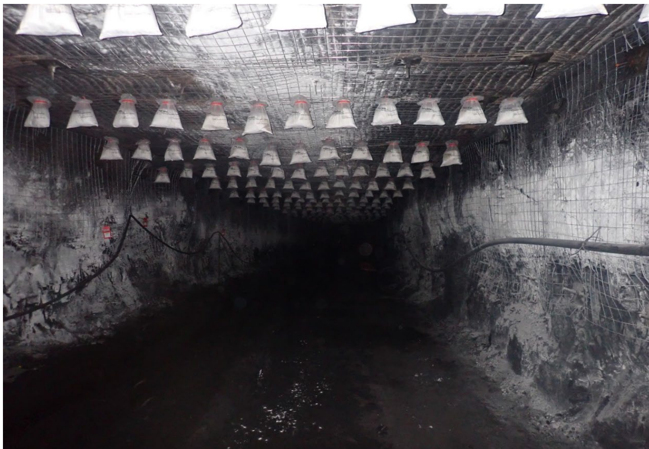
Image 5: Example of a high standard of installation of a Fixed concentrated barrier in an operational development panel face zone.
