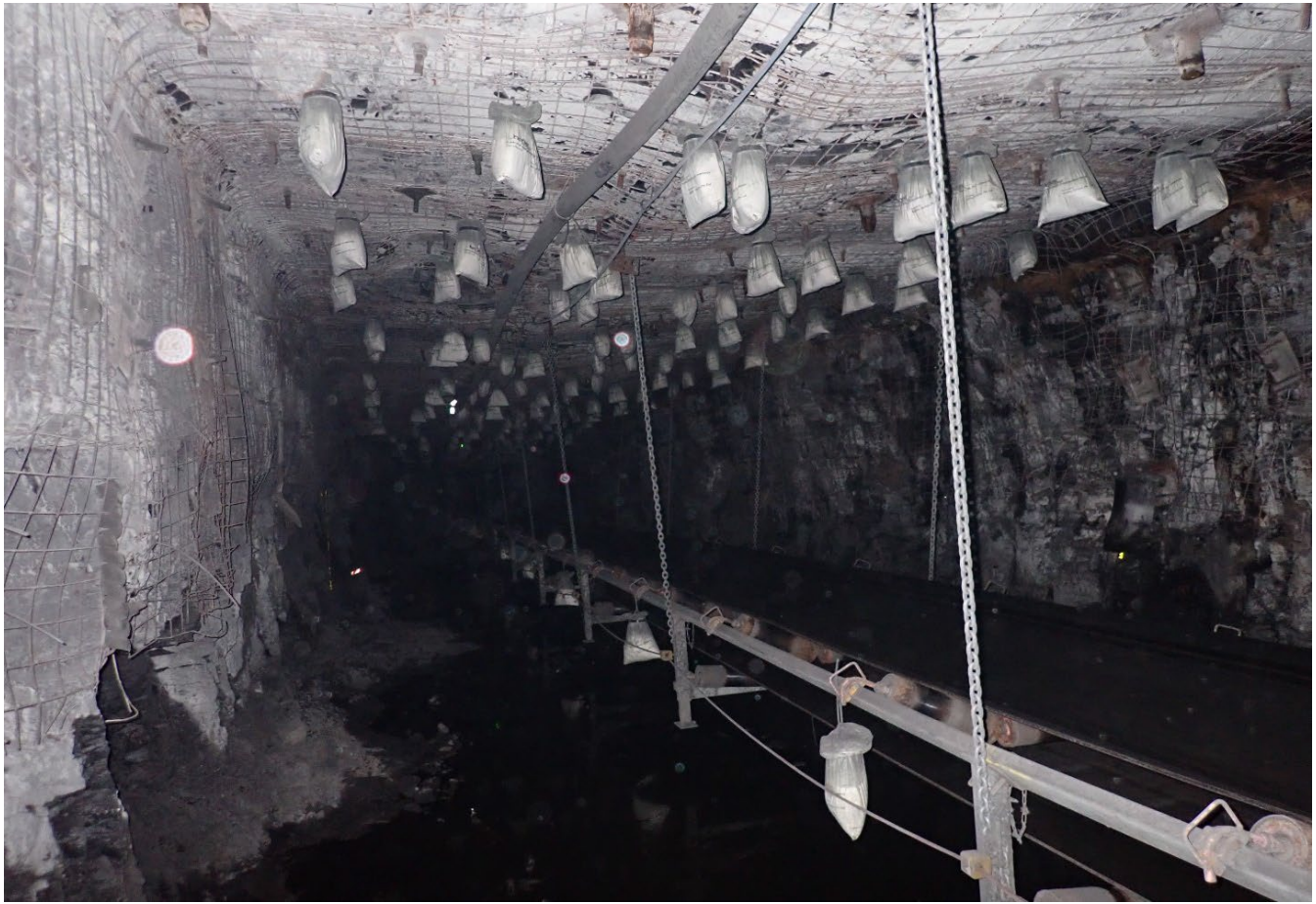
Image 7: Example of a poor standard of installation of a Fixed Continuous distributed barrier in an operational development panel face zone.
