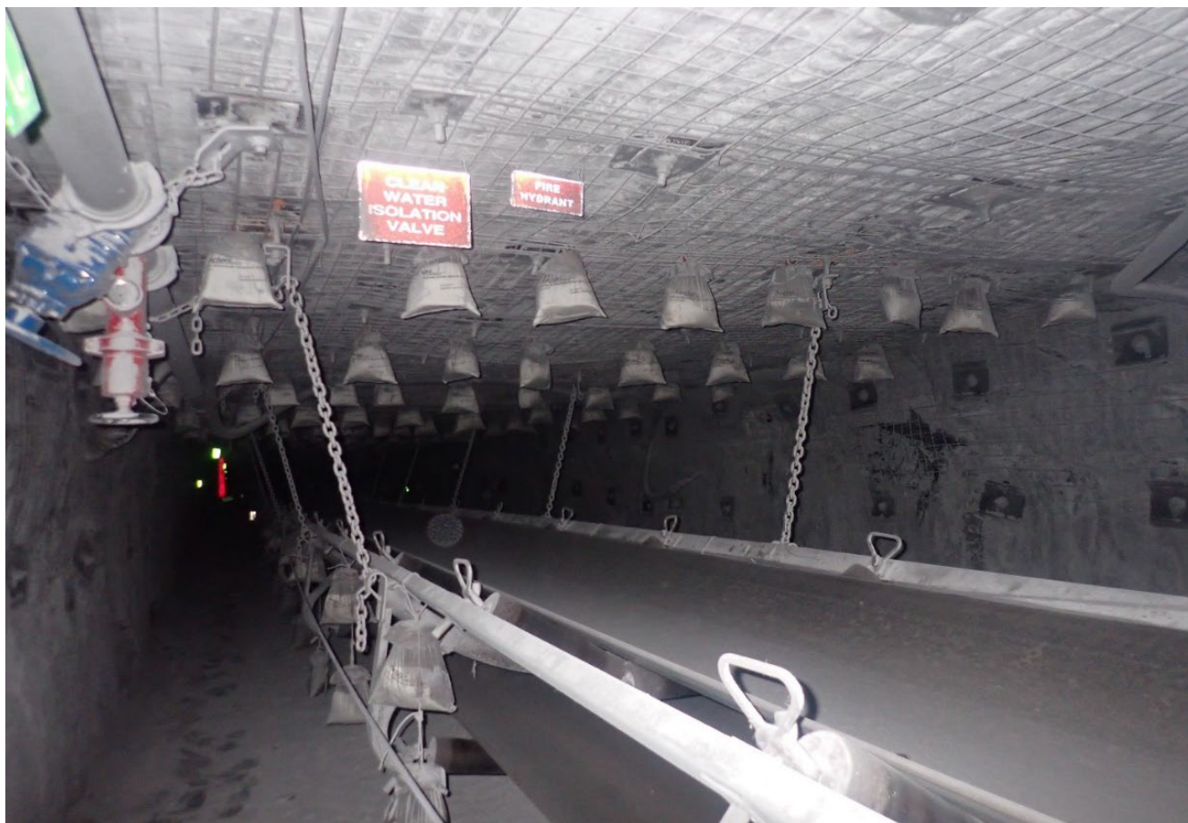
Image 4: Example of a high standard of installation of a Fixed Concentrated barrier in an operational development panel face zone.
