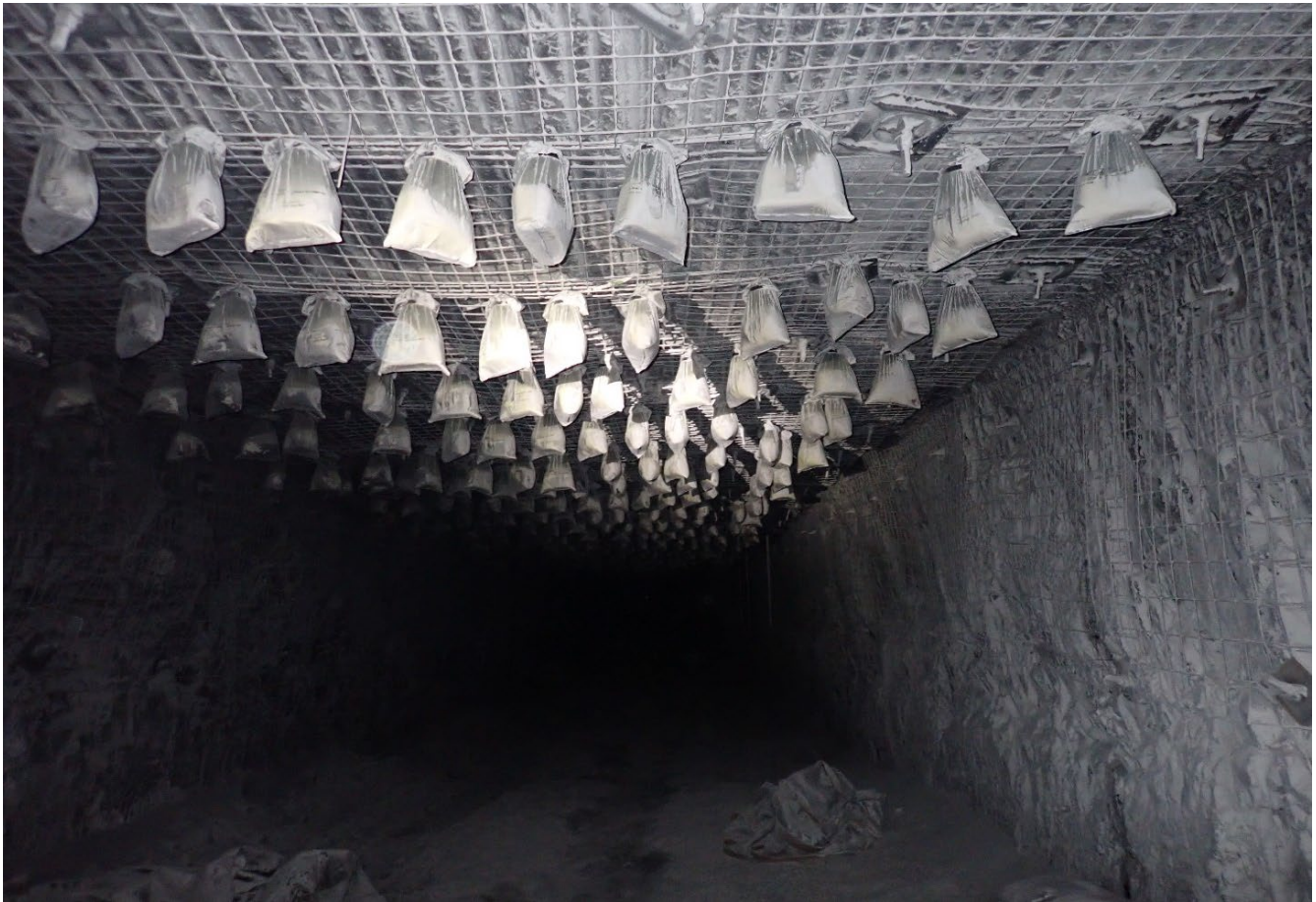
Image 6: Example of a poor standard of installation of a Fixed Concentrated barrier in an operational development panel face zone.
