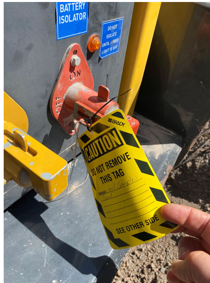
Caution tag applied - bad oil samples
