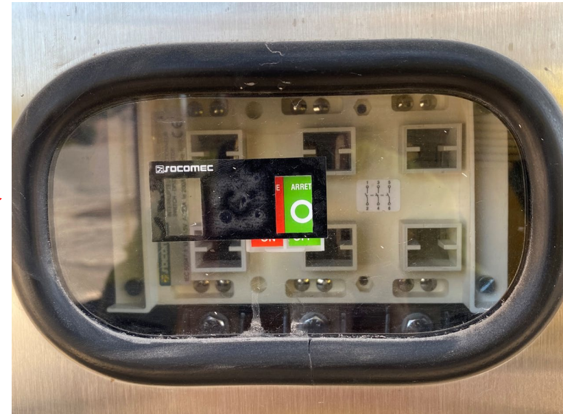
Visible break isolator
