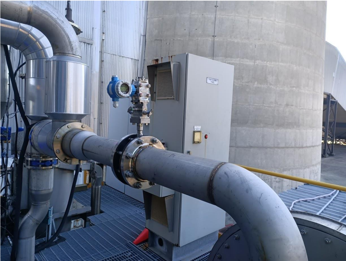
Figure 33 New flue gas flow meter
