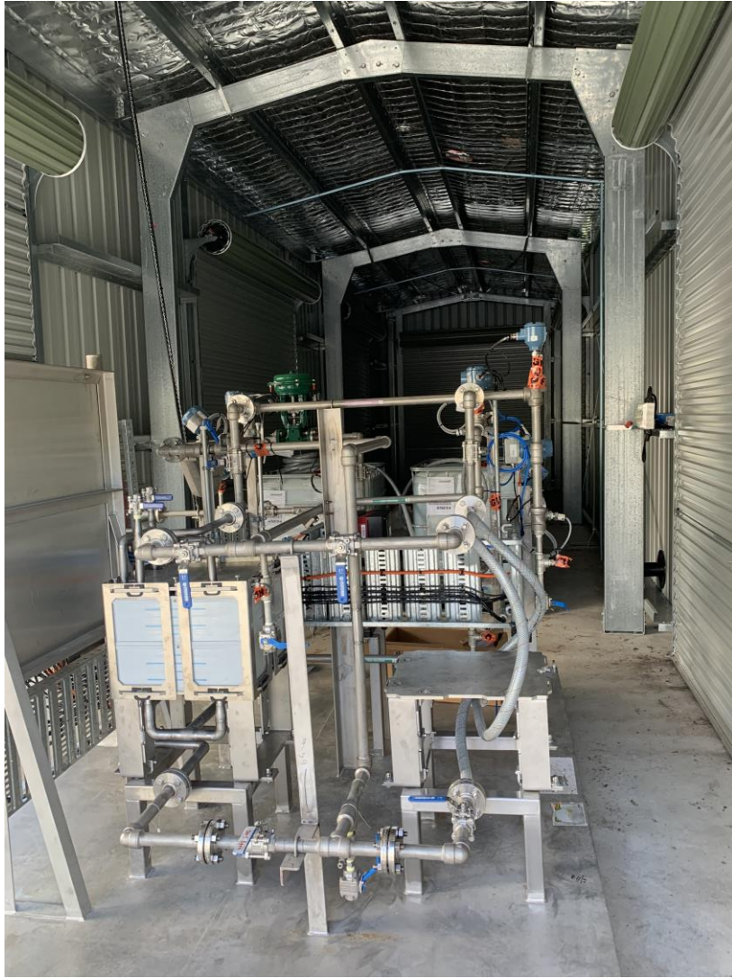
Figure 48 Forward Osmosis rig with half of membrane modules installed (left side of picture)
