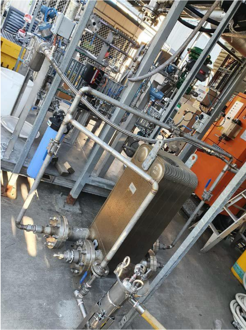
Figure 51 : Heater to control solution temperature to the Forward Osmosis unit
