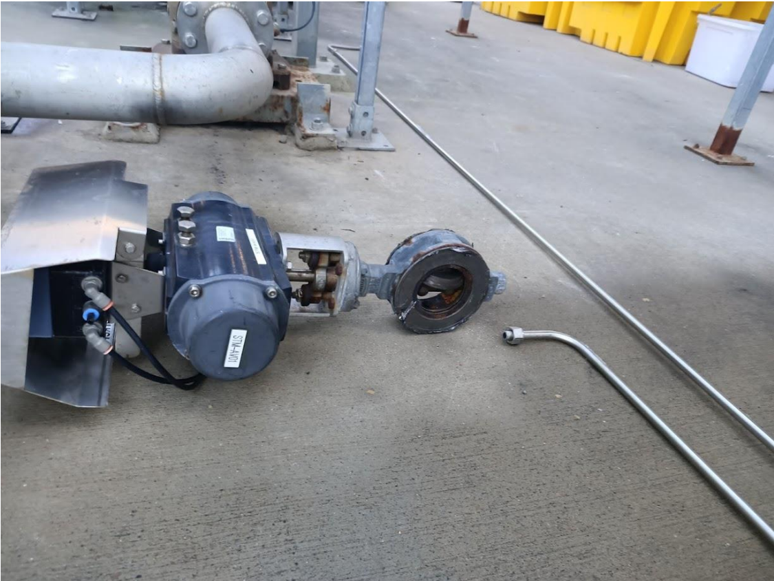
Figure 34 Damaged steam flow meter
