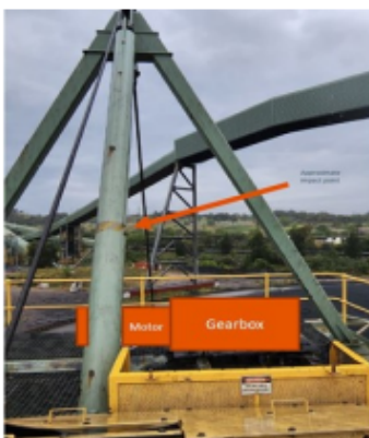
Figure 1: Reclaimer motor and gearbox
