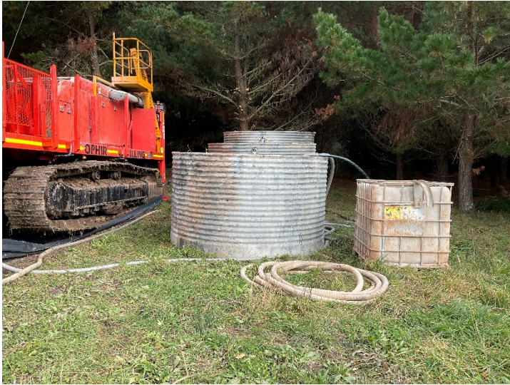
Figure 3 Above ground sumps for water management
