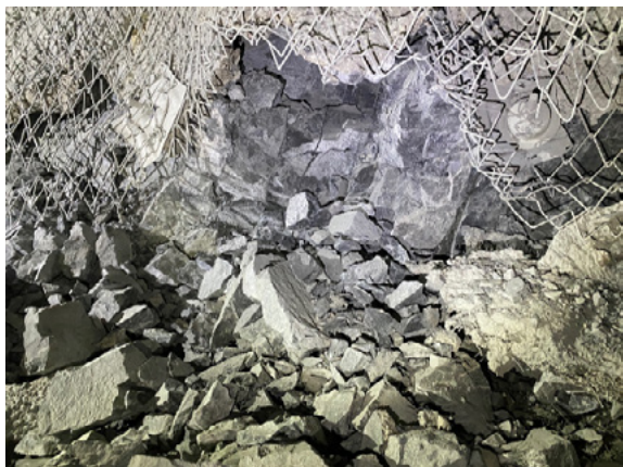
Picture 5. Rock burst.
