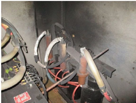
Picture 17. Result of arc fault.
