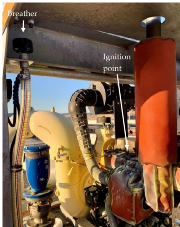
Picture 12. Ignition point on pump.
