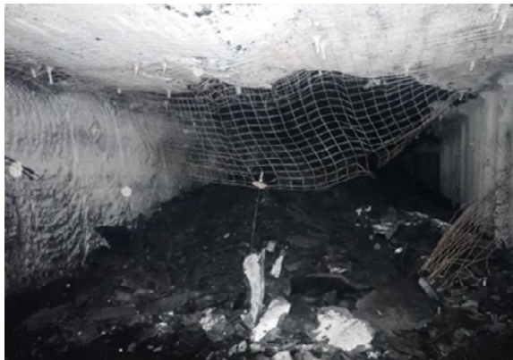
Picture 2. Extent of the fall debris.
