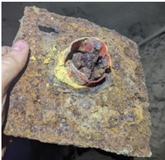
Picture 4. Close up of the corrosion damage.
