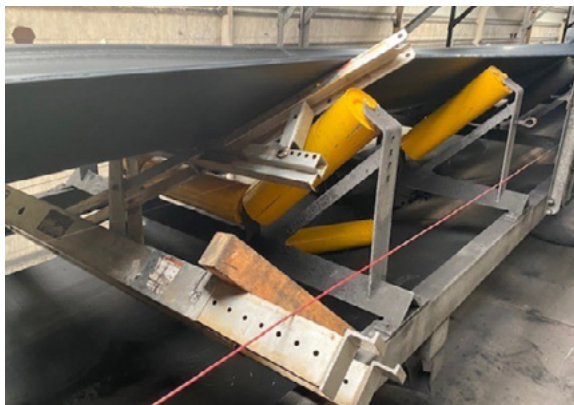
Picture 13. Showing lifters caught under the belt.
