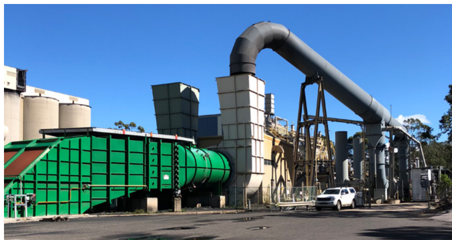
CSIRO VAMMIT technology deployed at Illawarra Metallurgical Coal operations to reduce fugitive emissions from coal mining.
