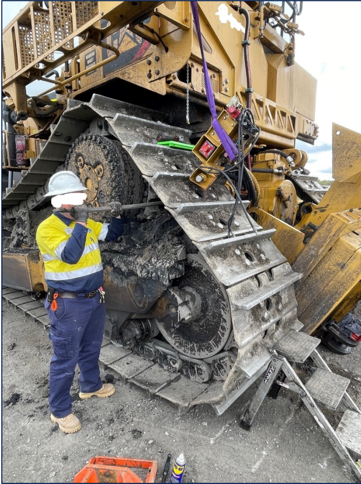
Figure 3 Post-incident simulation of the injured worker and position of the crowbar under the dozer track to push the second top securing pin horizontally so as to release the counterweight
