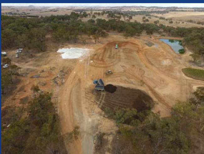
Kangiara Mine before remediation and rehabilitation works, March 2017
