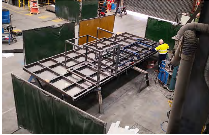
Figure 47. A photograph of the base metal structure of the furnace unit being built.
