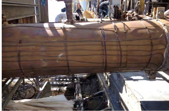
Figure 9 Electric heat tracing system in a molten salts pipeline (source: Abengoa)
