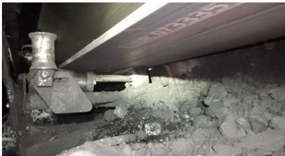
Below: Coal build up under the belt.
