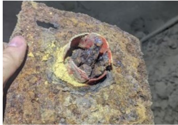
Below: Close up of corrosion damage.
