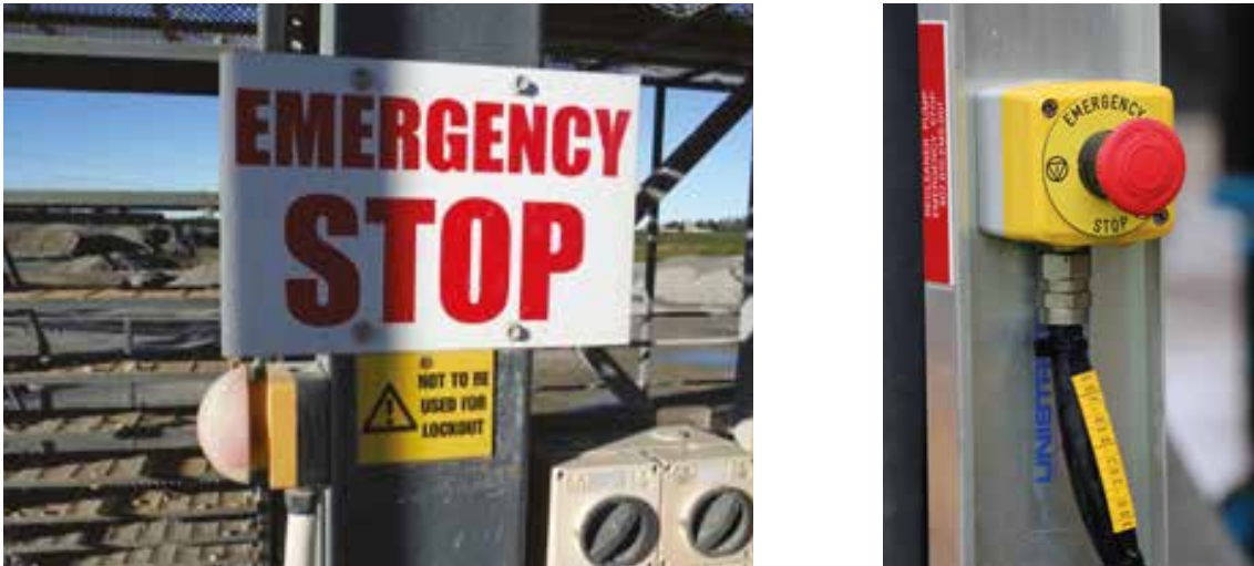
Figure 91. Emergency stop with signage (photo courtesy of Fulton Hogan Miner Rd Quarry and NZ Steel Taharoa)
