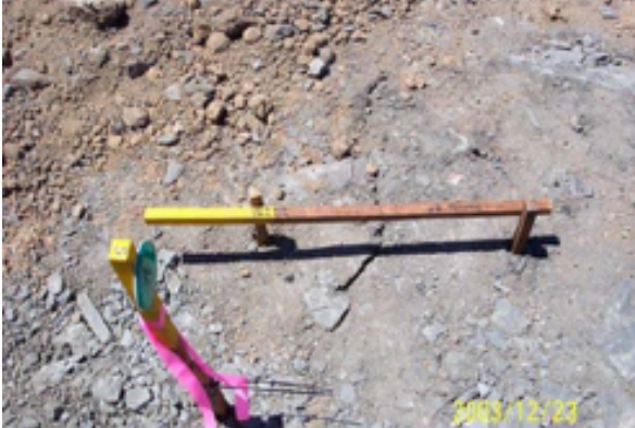
Figure 37. Measuring a ground crack that has opened up
