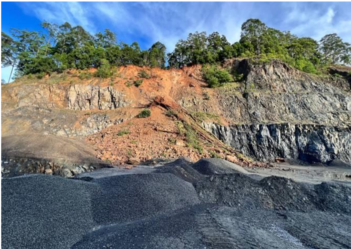
Figure 1: Failure of overburden bench.
