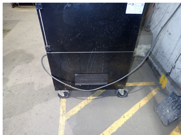
Figure 2: exhaust vent shown on side of unit.
