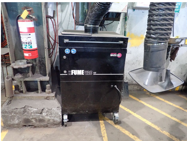
Figure 1: Typical portable LEV unit. (Note the snorkel hanging in the foreground)
